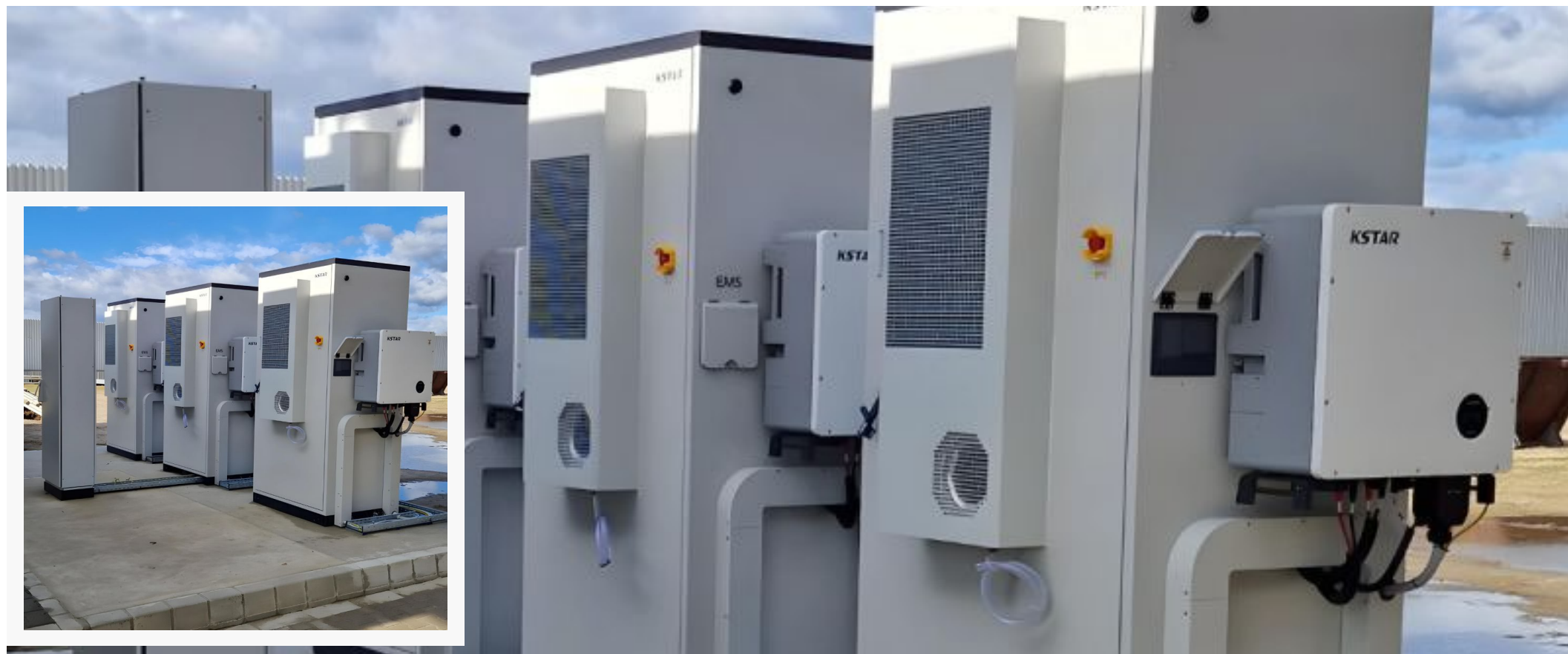
02 C&I ESS Project in the Netherlands
