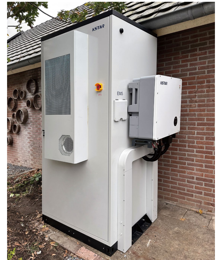
03 C&I ESS Project in Hungary
